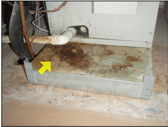
Stains indicate previous leakage
