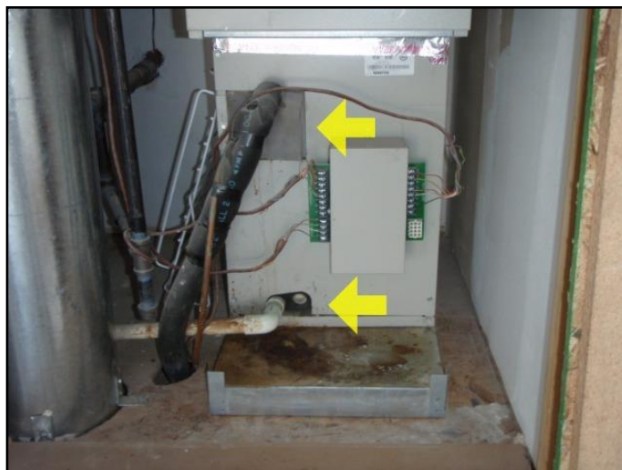
Locations of air leakage
