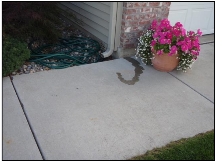
Downspout discharges at foundation
