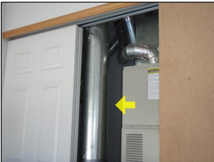
Non-insulated duct in garage
