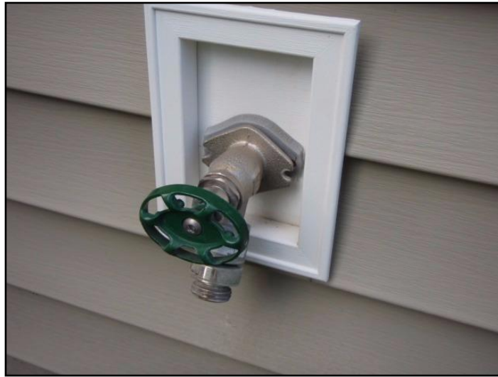
Hose faucet is loose from wall
