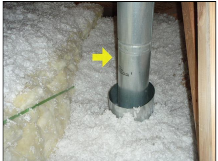
Water stains on vent pipe in attic
