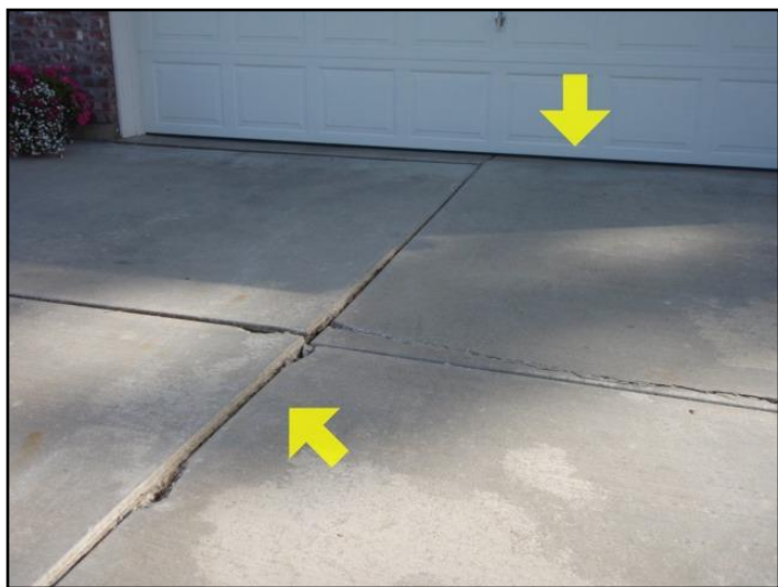
Trip hazards on the driveway
