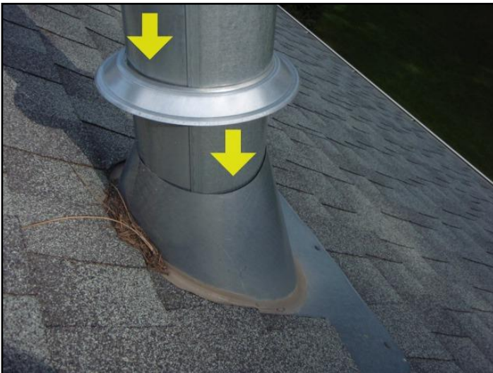
Gaps at the storm collar
