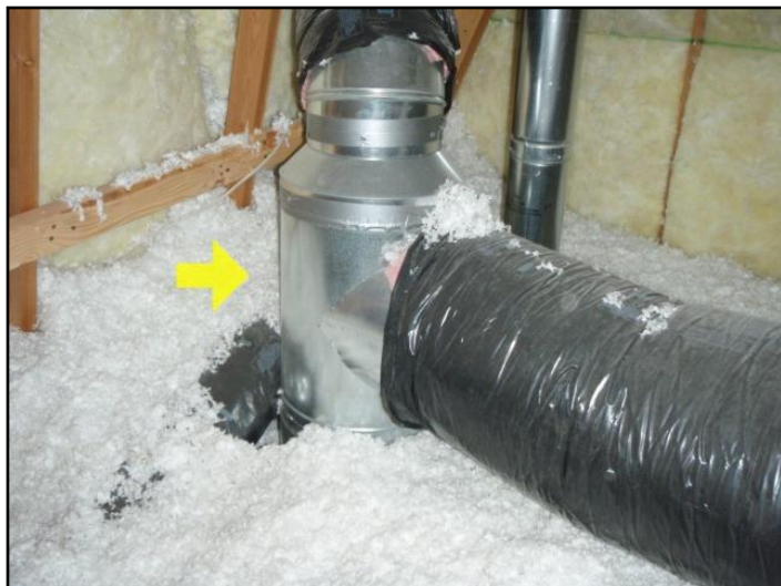
Non-insulated duct in attic
