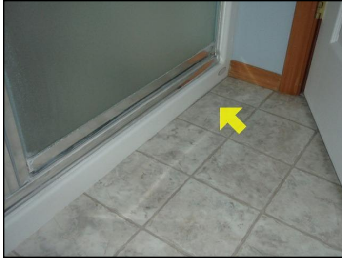
Vinyl flooring is loose at shower
