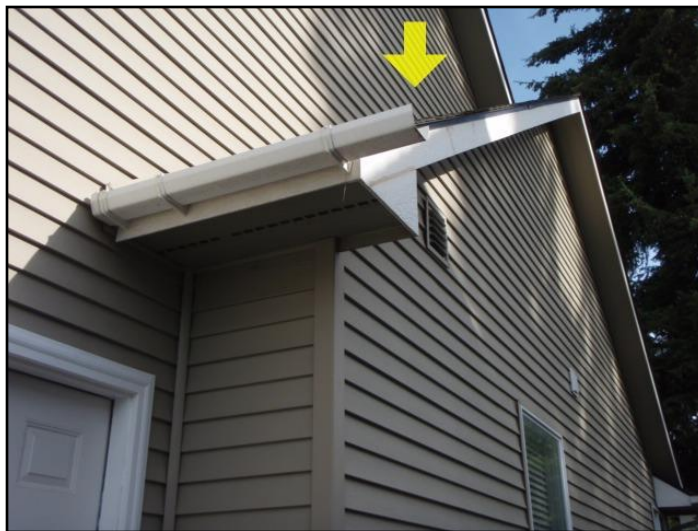
Missing downspout at gutter
