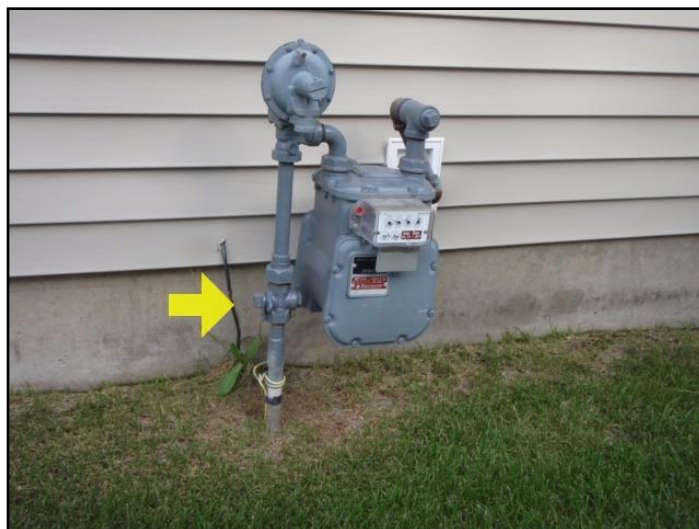
Main gas shut-off valve
