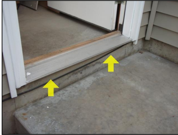
Metal threshold is poorly supported
