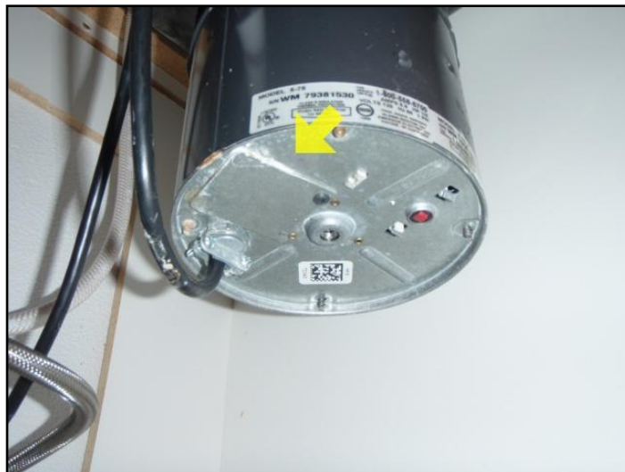
Leak at disposal
